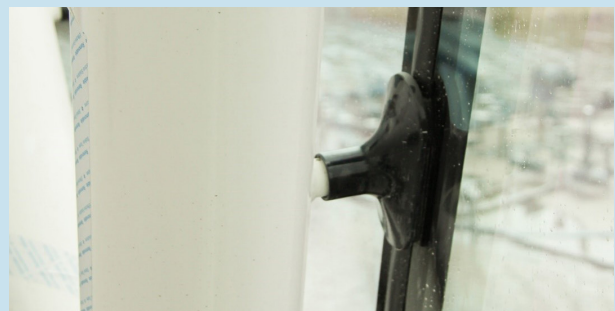
Figure 2: A support to visually disconnect the glass skin from the main steel structure
