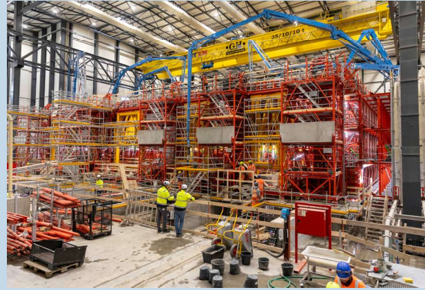
Figure 3: In the summer of 2023, the first tunnel element segment was casted (Photo: Femern A/S)
