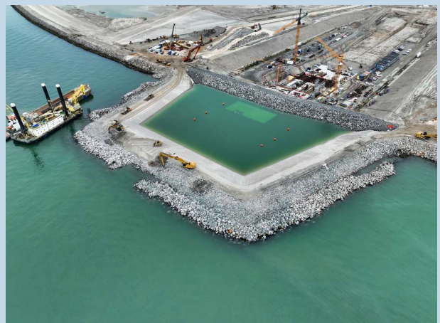
Figure 7: Outer retaining dike removal on Lolland, the tunnel portal is visible underwater (Photo: Femern A/S)
