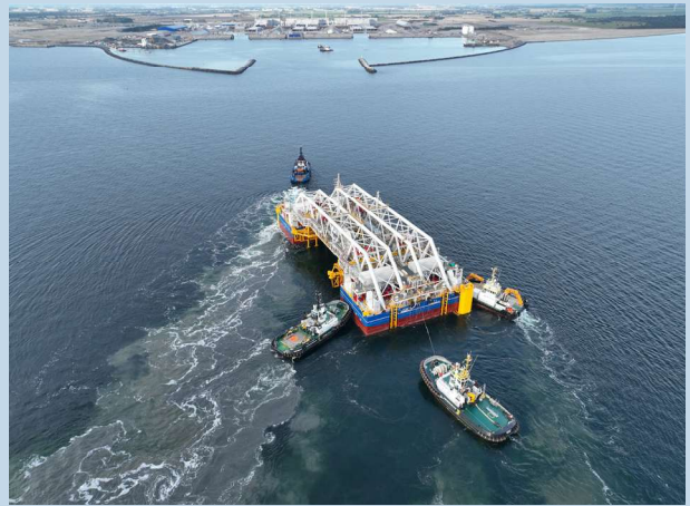
Figure 6: Immersion pontoon IVY arrives in September 2024 in the working port of Lolland (Photo: Femern A/S)
